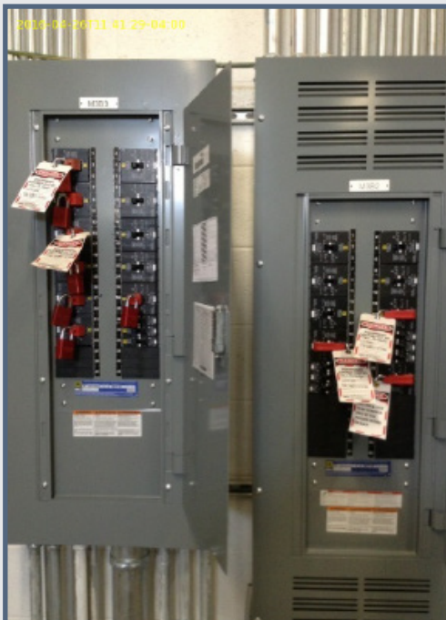
Single Lock and Tag on Each Breaker
