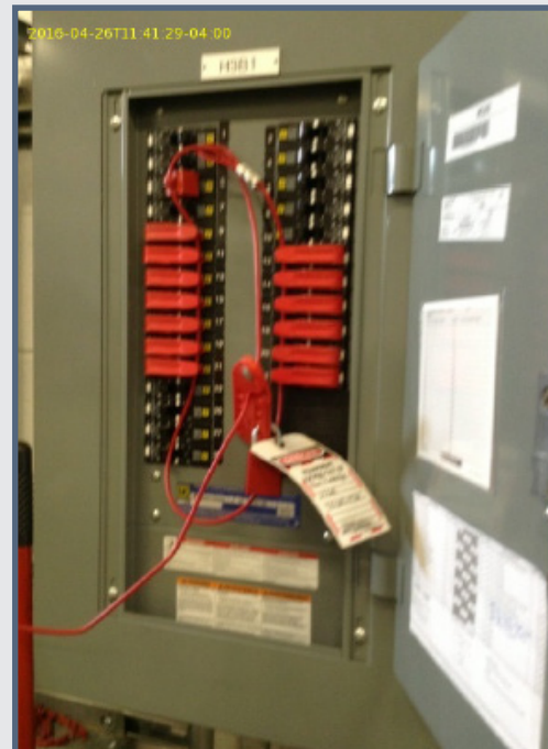
Cable Lock Out passed through multiple breakers with one lock
